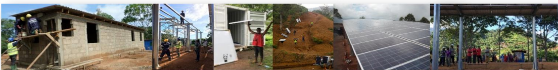
2017: ENSOL & TTA: Design, Construction, and O&M of 1 Solar PV micro-grids (48 kWp) in Mpale, TZ
